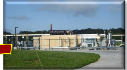
CNG compression plant
