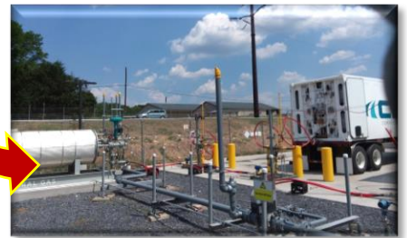
CNG customer delivery pad
