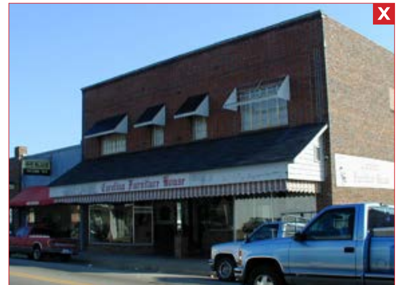
Shingled canopy appears as oversized awning concealing transom, sign panel & upper façade components.
