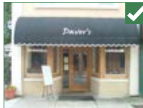
One way to deal with the transom area is to conceal it with an awning. All the other elements of the traditional storefront are dealt with appropriately in this example.
