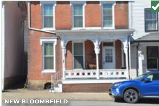
Decorative foundation vents on this building provide ventilation to the sub-floor area.
