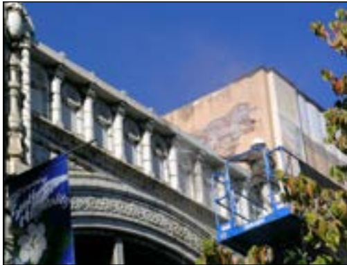
Terra cotta cornice cleaning via a low-pressure water wash and mild detergent.
