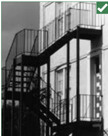
The placement of fire escapes at the rear of buildings usually is appropriate.
