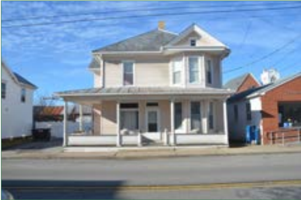
Some disadvantages of vinyl siding placed over wood siding include, but are not limited to: the concealment of any deterioration issues; corner trims and window surrounds that are not sized appropriately; and, an appearance that is "too perfect," and therefore, doesn't look authentic.
