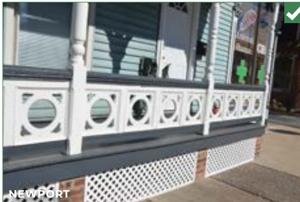
Wood lattice placed between brick foundation piers provides ventilation to the crawl space.
