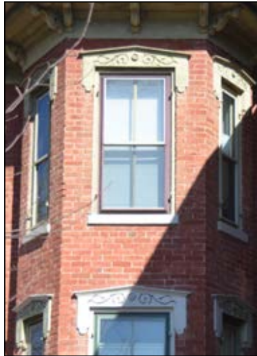
The name “window” is derived from a word that literally means “wind’s eye”—indicating the fact that windows at one time were only shuttered openings. Casement windows are a type that predates sash windows.
